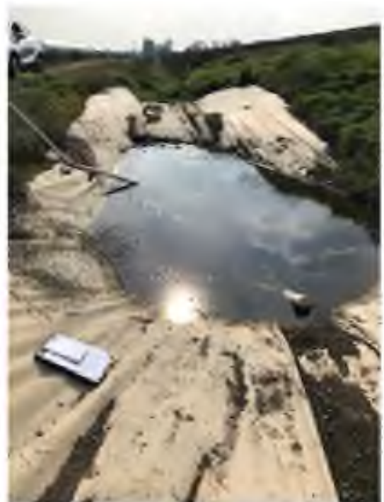
Subsidence since repair (~12 years and 1.5 ft depth)
