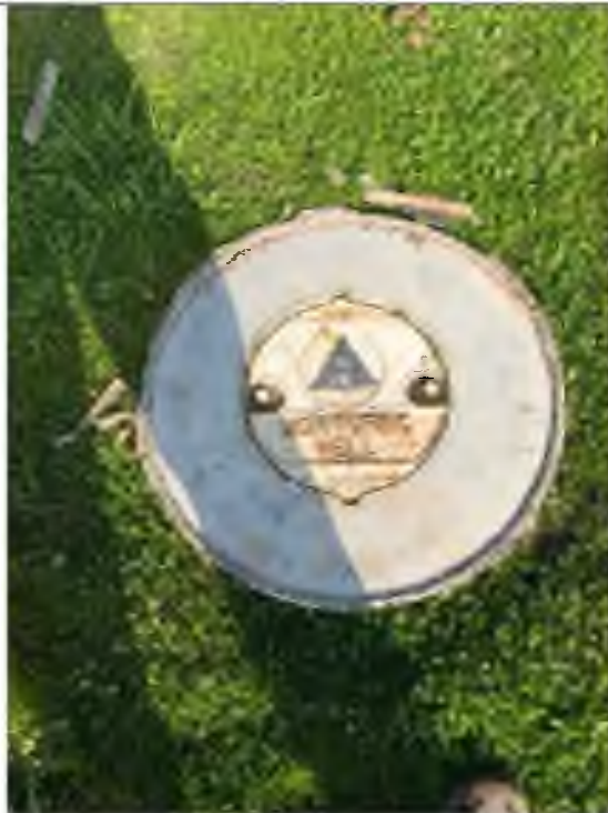
Monitoring well PZ-10
