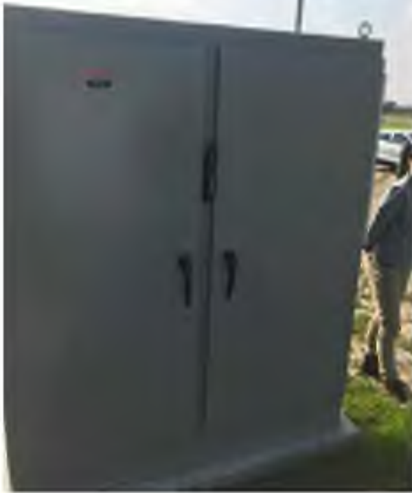
Extraction well electrical panel
