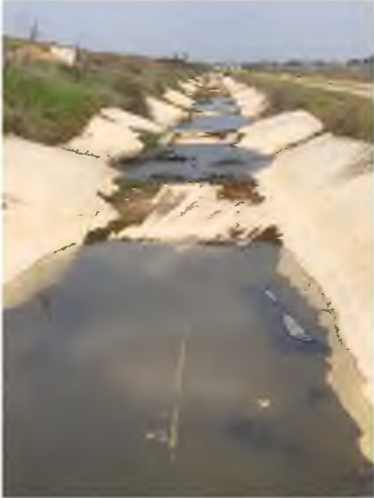
Subsidence in drainage ditch
